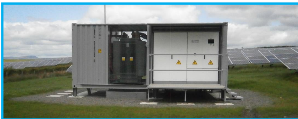
Fig 4 Typical cabin mounted transformer on permeable gravel (Merthyr Tydfil).
